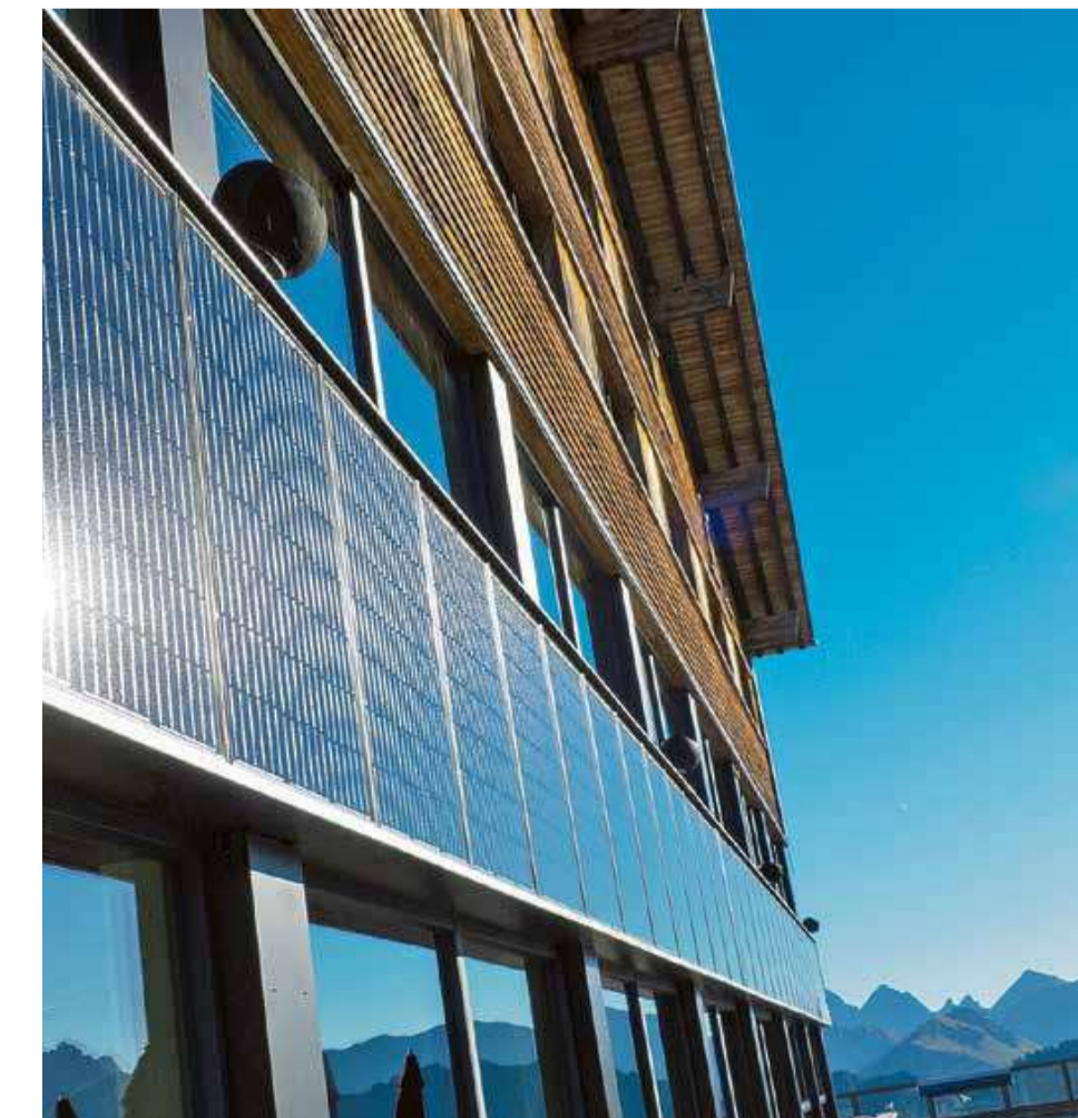
Photovoltaik-Anlage am Fellhorn
